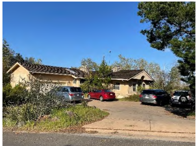
Exhibit 12. Wood shake roof on home along Altamont Road.
